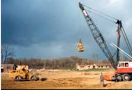
First deep dynamic compaction performed for Bob Evans project in South Columbus.
